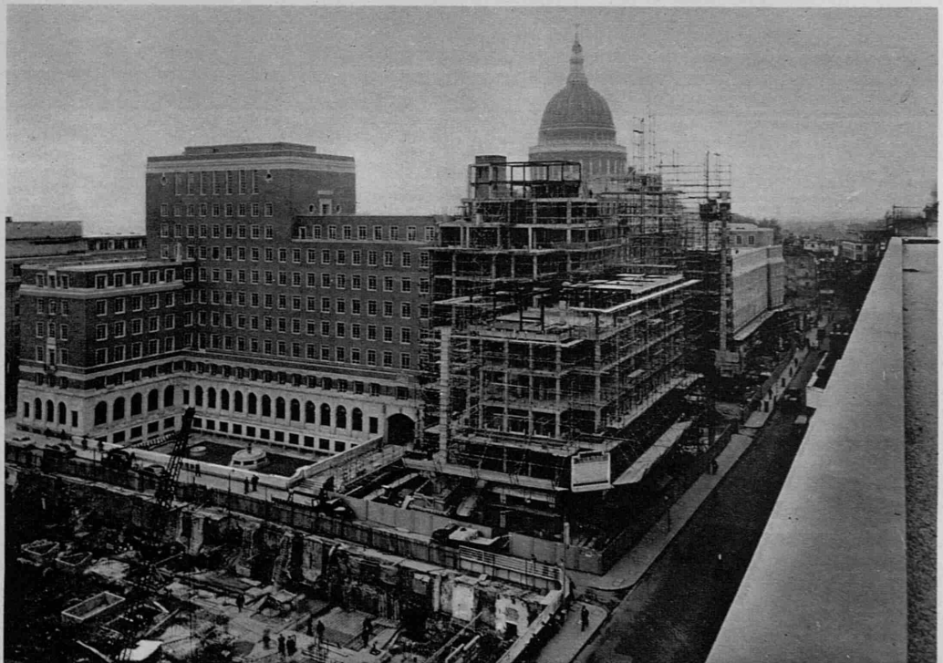
REBUILDING IN THE CITY OF LONDON: The new Bank of England building, close to St. Paul's Cathedral, is under construction by Holland & Hannen and Cubitts. It is a steel-framed building with brick cladding, and is faced with Portland stone. The architect is Victor Heal. The Cubitt group of companies is taking a prominent part in the rebuilding of the City.
